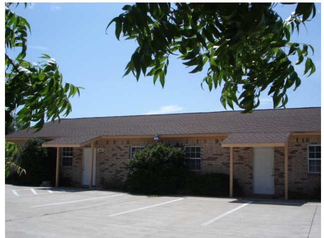
A new roof was added in early summer in addition to protective porches over the two front entrances.
